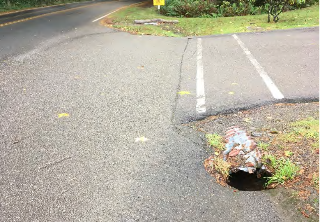
Failed culvert on Scenic Drive (exposed end is a hazard to vehicles)
