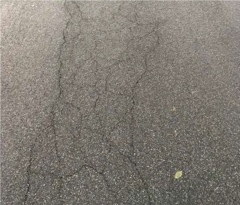
Severe alligator cracking/rutting (pavement failure) on Trinity Street.
