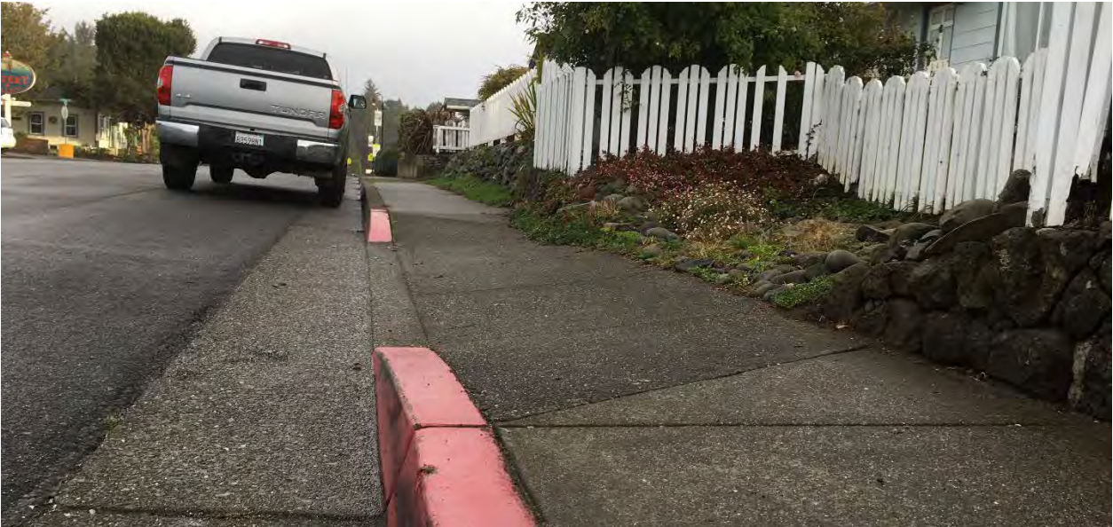
Example of non-accessible/non-compliant sidewalk on Trinity Street (cross slope >5%); Typical of 12 locations on Trinity Street.
