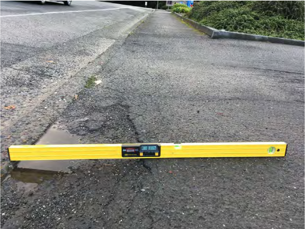
Non-accessible/non-compliant driveway on Patrick's Point Drive (cross slope 8.1%)
