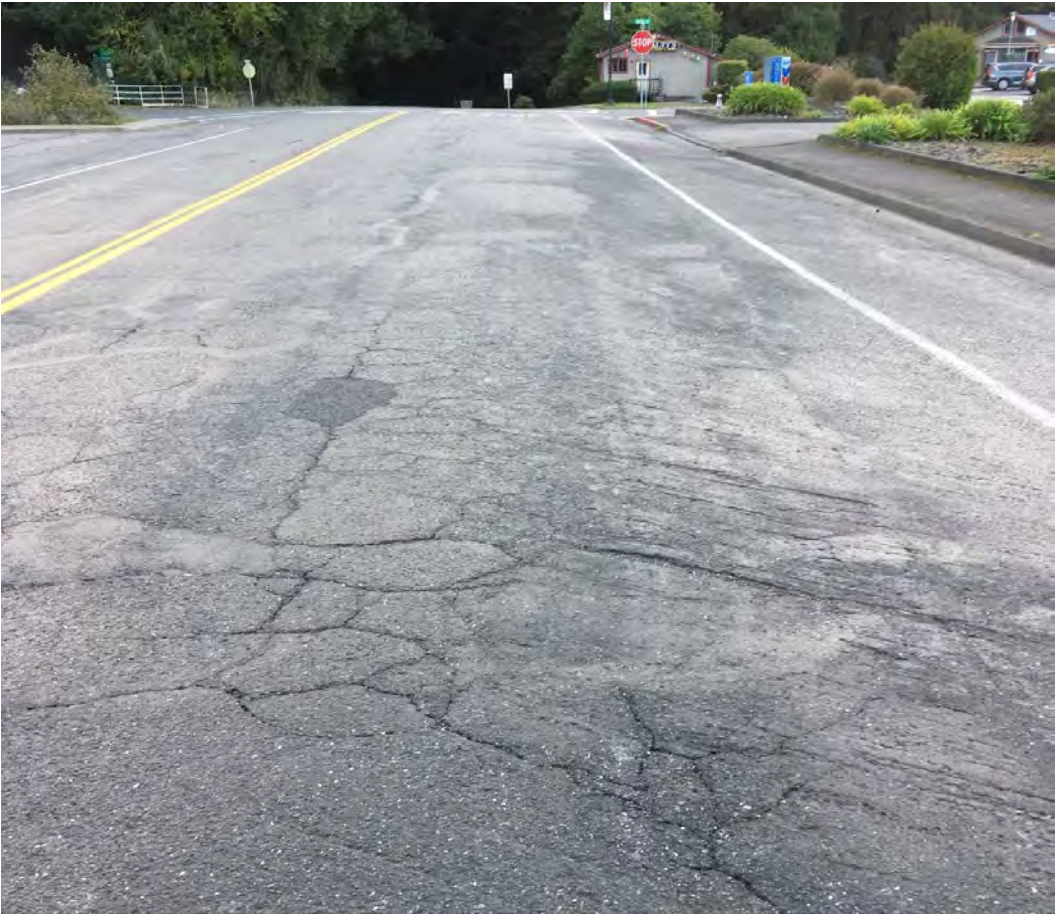
Severely failed pavement on Patrick's Point Drive.
