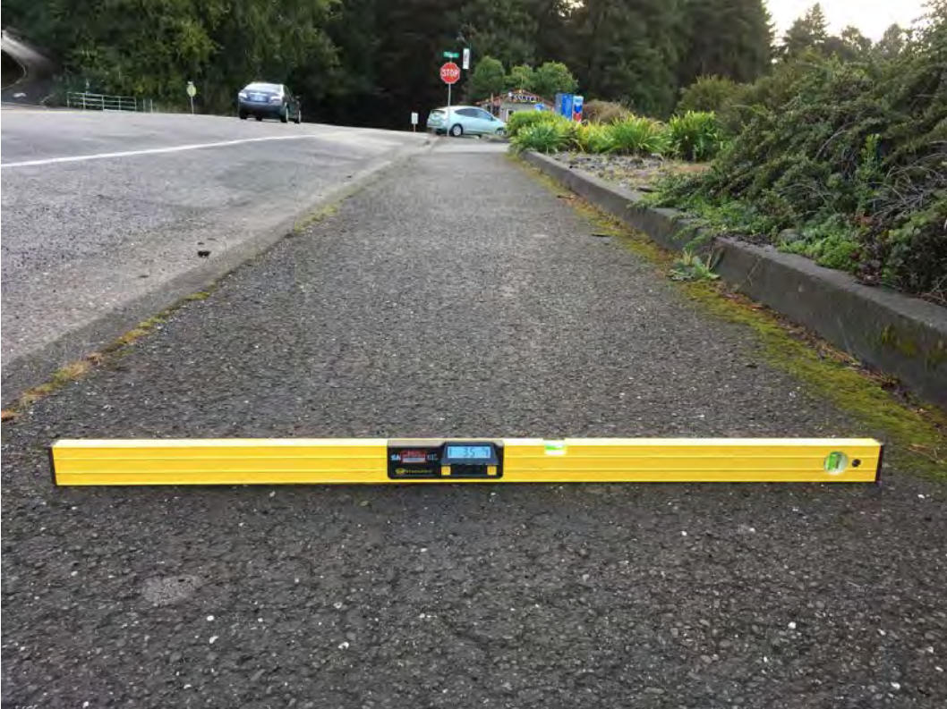
Non-accessible/non-compliant sidewalk on Patrick's Point Drive (cross slope 3.5%)
