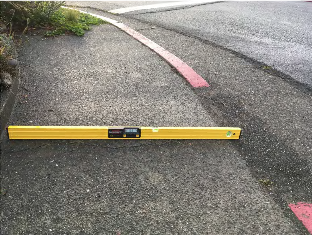
Non-accessible/non-compliant curb ramp on Trinity Street (cross-slope 6.3%); Typical of 6 locations on Trinity Street.
