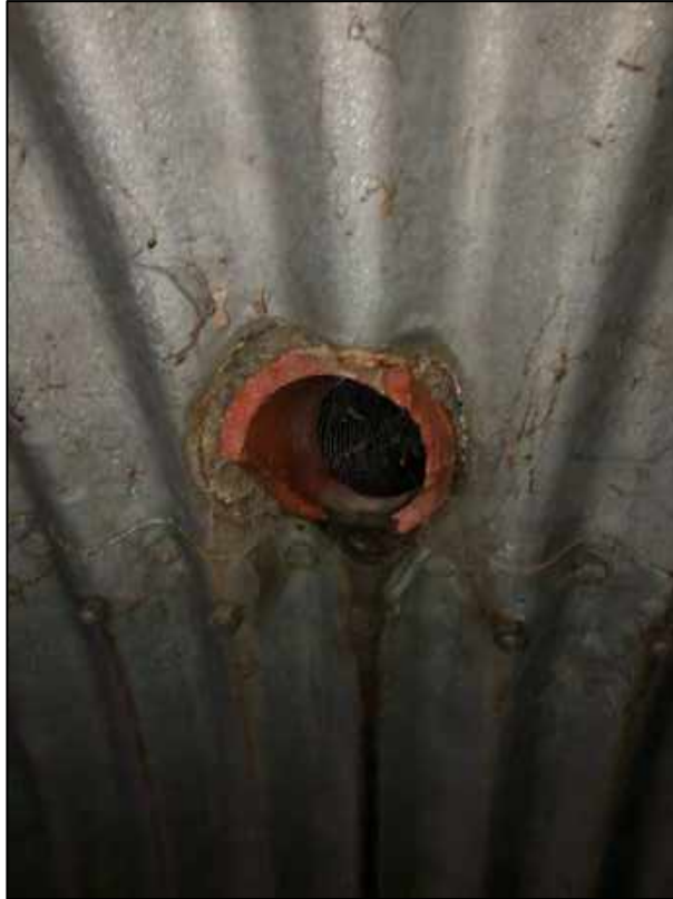
Photo 3. Outlet of VCP stubbed into CMP sidewall (Storm Drain Improvement #1)
