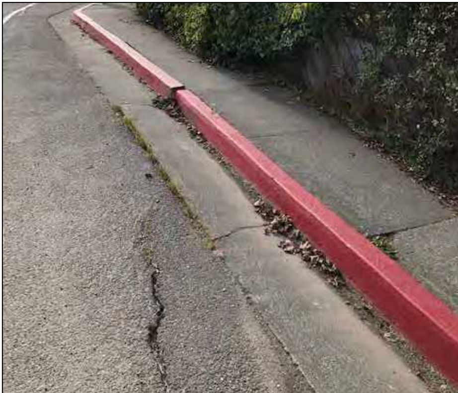
Photo 2. Surface Failure Along Alignment (Storm Drain Improvement #1)
