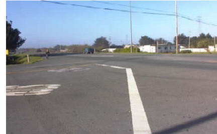
The long width and high speeds of SR 255 through Manila makes pedestrians crossings difficult.
