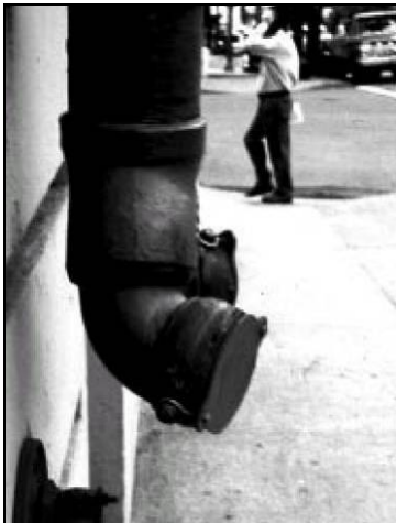
Elements such as standpipe systems may project into the Frontage Zone. Care must be taken to assure compliance with the ADA.
